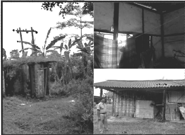
Figure 2 : Condition of a quarter for staff-members of the Jorhat District Jail. Left- Toilet. Right- Interior and exterior of the quarter. (Source: Pratidhwani: Free Legal Aid and Awareness Centre)
