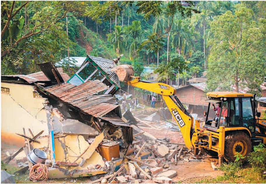
Houses in Amchang Wildlife Sanctuary were demolished as part of a November 2017 eviction drive. (Photo credit: Kuntala Roychudhury.)
